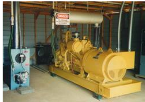
Photo of a 120kW engine generator set combusting recovered biogas, generating electricity for on-farm use 6
